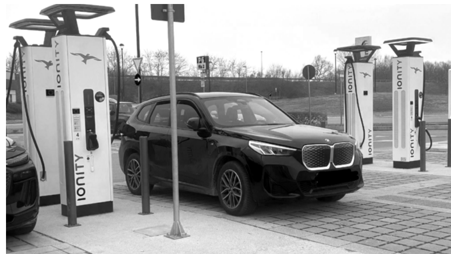
EV charging station in Mondovì (CN)
